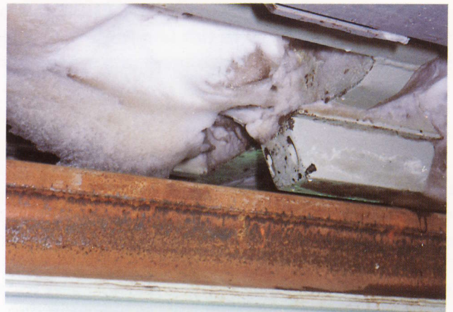
Status of track displacement sensor when frozen
