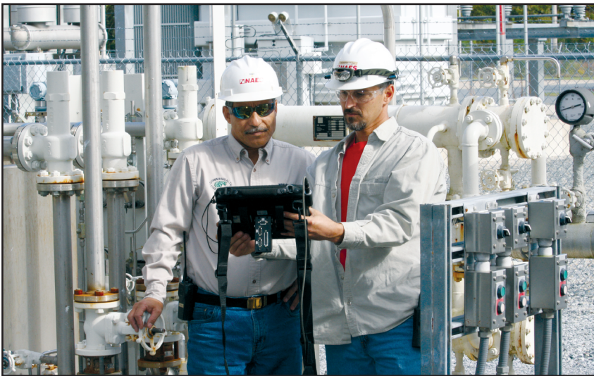
Commonwealth Chesapeake operators reviewing vibration data on one of the plant's generator lubricating oil pumps.
