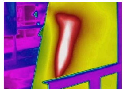
Vessel Refractory Failure
