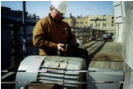
Figure 5. Portable Collection of Vibration Data from Cooling Tower
